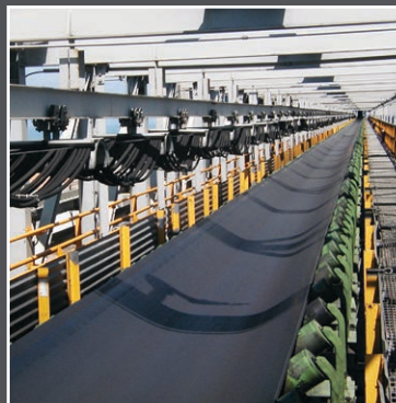
Festoon System on a Tripper Conveyor, Venezuela
