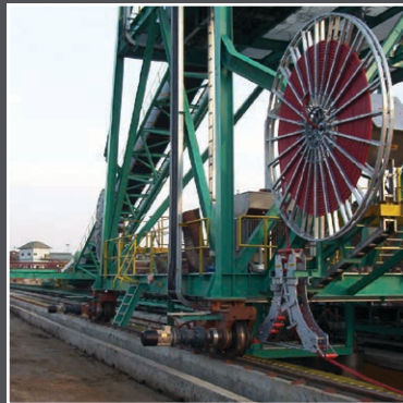
Motor Driven Cable Reel on a Stacker/Reclaimer, Thailand
