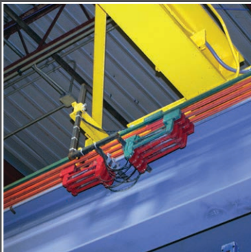
Conductor Bars on an EOT Crane, USA
