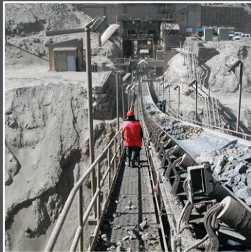
Festoon System on a Conveyor, Chile
