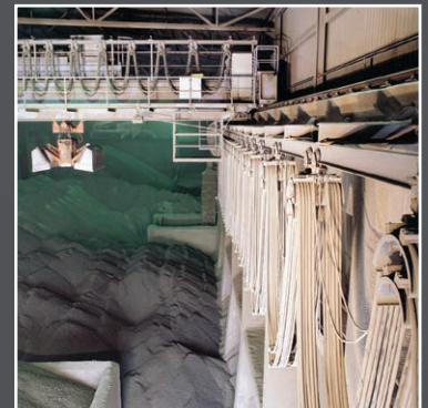
Festoon System on a Bridge Crane with Grab, Germany
