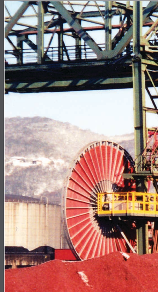
Motor Driven Cable Reels on a Ship Unloader, Germany
