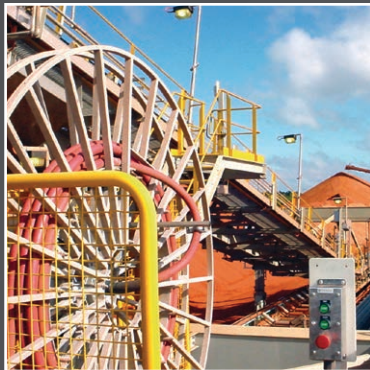
Motor Driven Cable Reel on a Stacker, Australia
