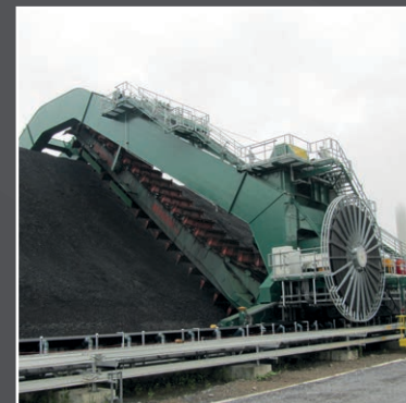
Motor Driven Cable Reel on a Portal Stacker, USA
