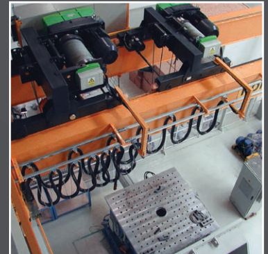
Festoon System on an EOT Crane, Czech Republic
