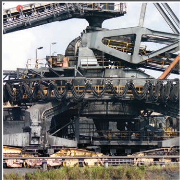
Festoon System on a Stacker/Reclaimer, Australia
